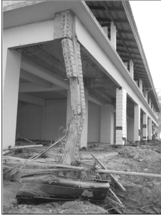
Figure 1.1: Damage caused by buckling in the column.
