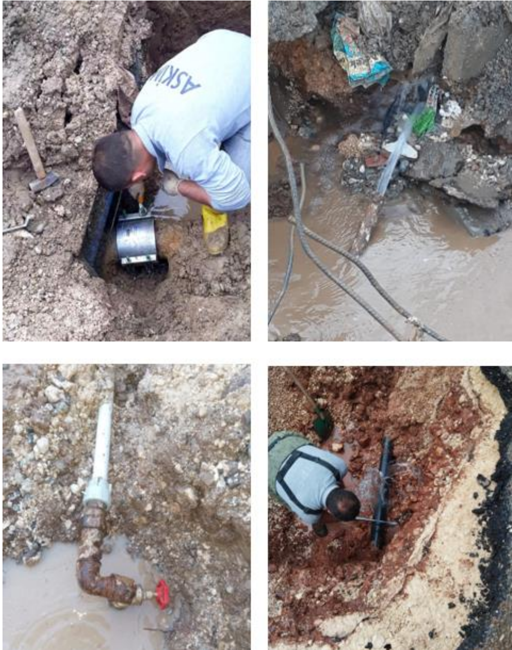
Figure 6.11: Some examples from distribution line problems in Adıyaman city center (ASKİM personal communication).
