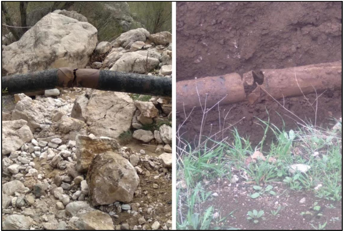
Figure 6.7: Damages in steel section of Gürlevik 1 transmission line.
