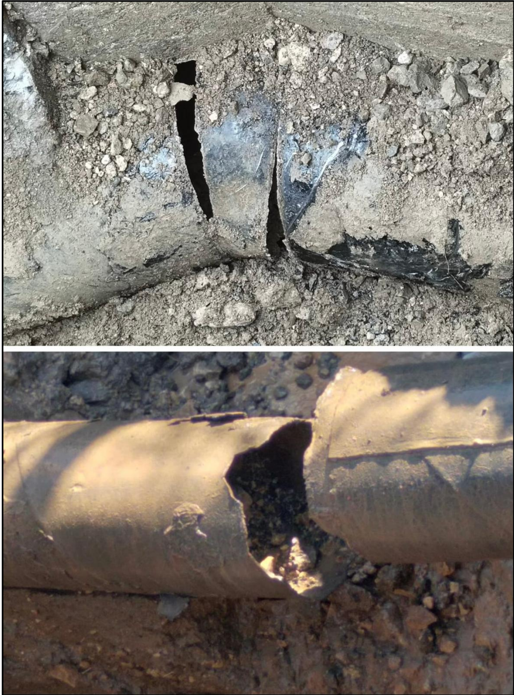
Figure 6.6: Damages in Gürlevik 2 transmission line.
