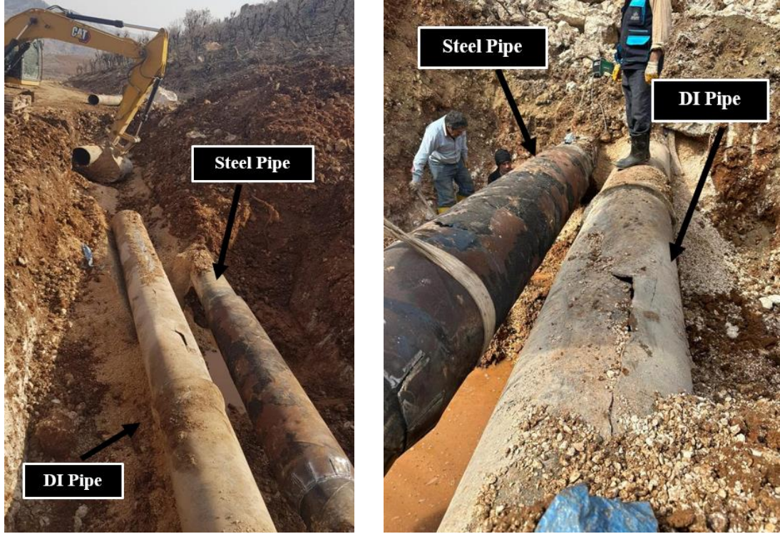
Figure 6.8: Damages in Gürlevik DI and 2 transmission lines due to rock falls.
