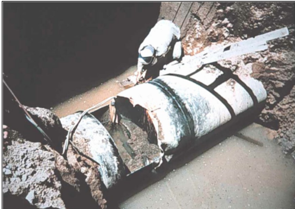
Figure 4.1: Failure of buried potable water pipes during 1985 Mexico City earthquake.
