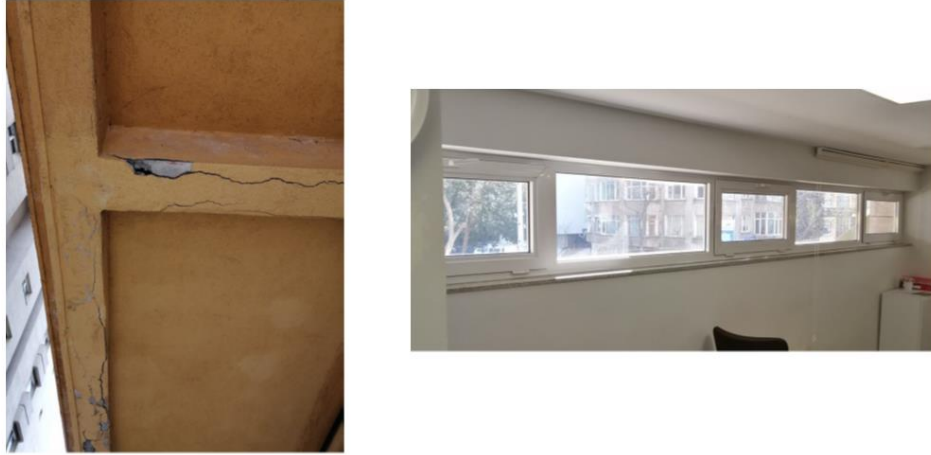
Figure 3.3: Possible corrosion indicators and short column effects.
