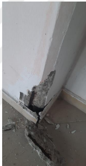
Figure A.15: Spalling and severe reinforcement corrosion
