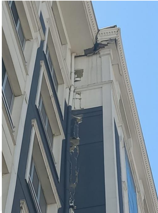
Figure 2.27: Examples of exterior nonstructural falling hazards.
