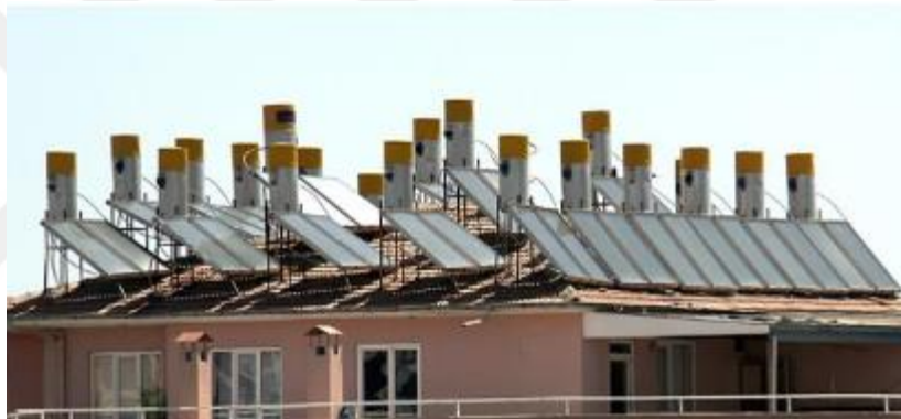
Figure 2.20: Solar panels with a risk of falling during an earthquake.
