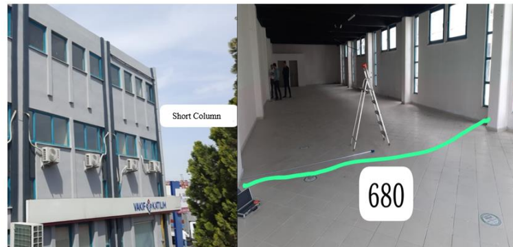
Figure A.14: Photos from structure (irregularities)
