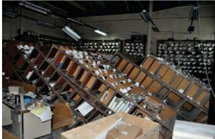
Figure 2.28: Examples of nonstructural hazards observed in interior spaces.
