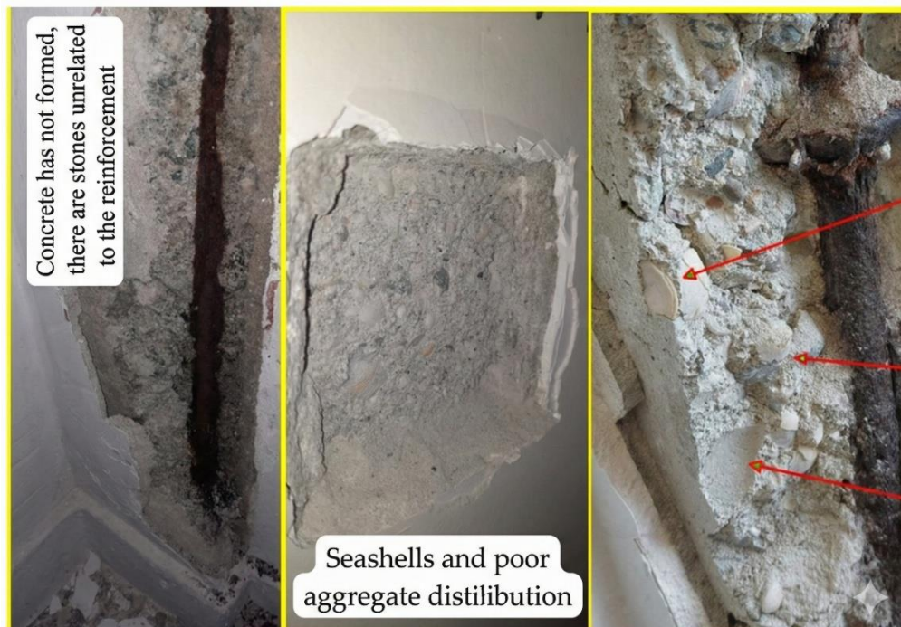
Figure 3.7: Concrete samples with irregular aggregate distribution.
