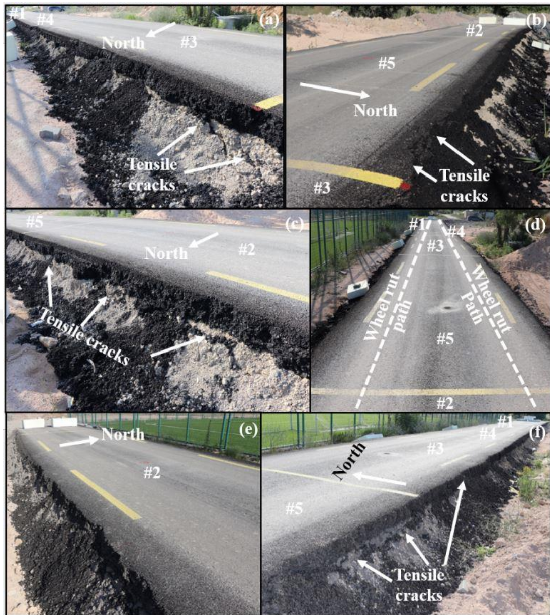
Figure 6.23: Physical conditions of Configurations #3, #5 and #2 at the end of the APT , a-c) Tensile cracks at configurations and HMA yielding towards to the slope-side of the pavement, d) Wheel rut path, e-f) HMA in the safety zone of configurations yielding and spreading along the slope-side.
