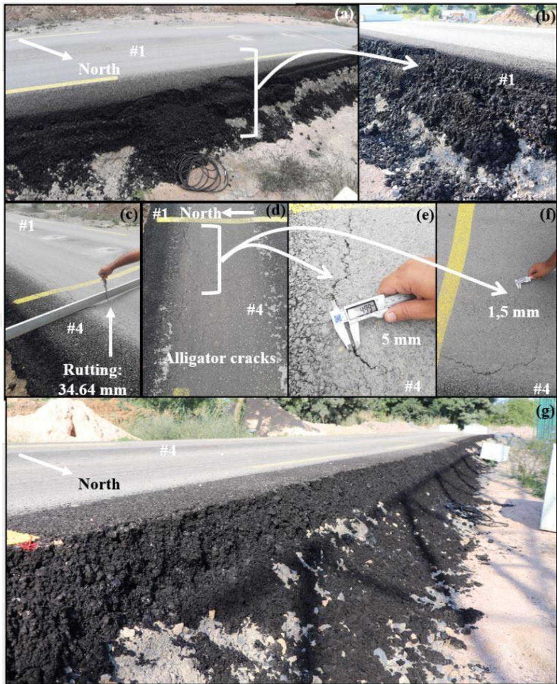
Figure 6.22: Physical conditions at the end of the APT test for Configurations #1 and #4, a-b) Tensile cracks at the crest of the northern safety zone of the Configuration #1 and HMA yielding towards to the slope-side, c-f) Rutting path of Configuration #4 and alligator cracks at the north-west of the Configuration #4, g) HMA in the safety zone of Configuration #4 were yielded along the northern slope-side of the pavement.
