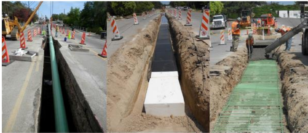
Figure 3.4: EPS slot-trench light-weight cover system constructed across the Wasatch fault in Salt Lake City, Utah [Bartlett et al., 2015].
